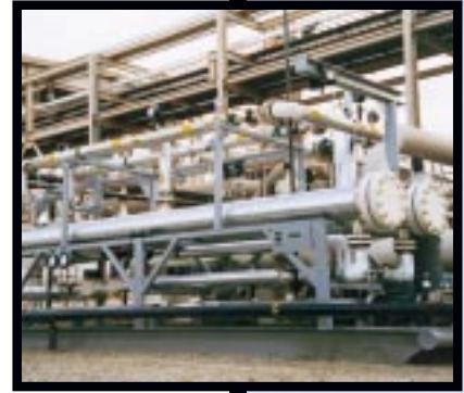
VaporSep system for LPG recovery.
