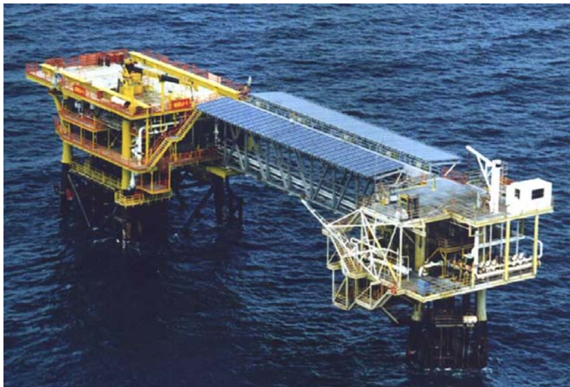
Eex Zone 1 certified solar power generator for a unmanned platform in the South China Sea. Load = 2.71 kW continuous, area of the modules = 300 m 2
