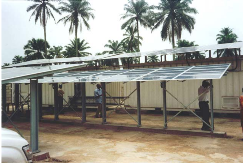
A Cathodic Protection system installed in West-Africa. Controllers and batteries installed in a 40 foot isolated seacontainer. Load =1200 W continuous.
